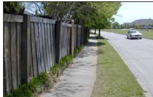
Illustration 5-17 Wood Screening Wall in Deteriorating Condition
