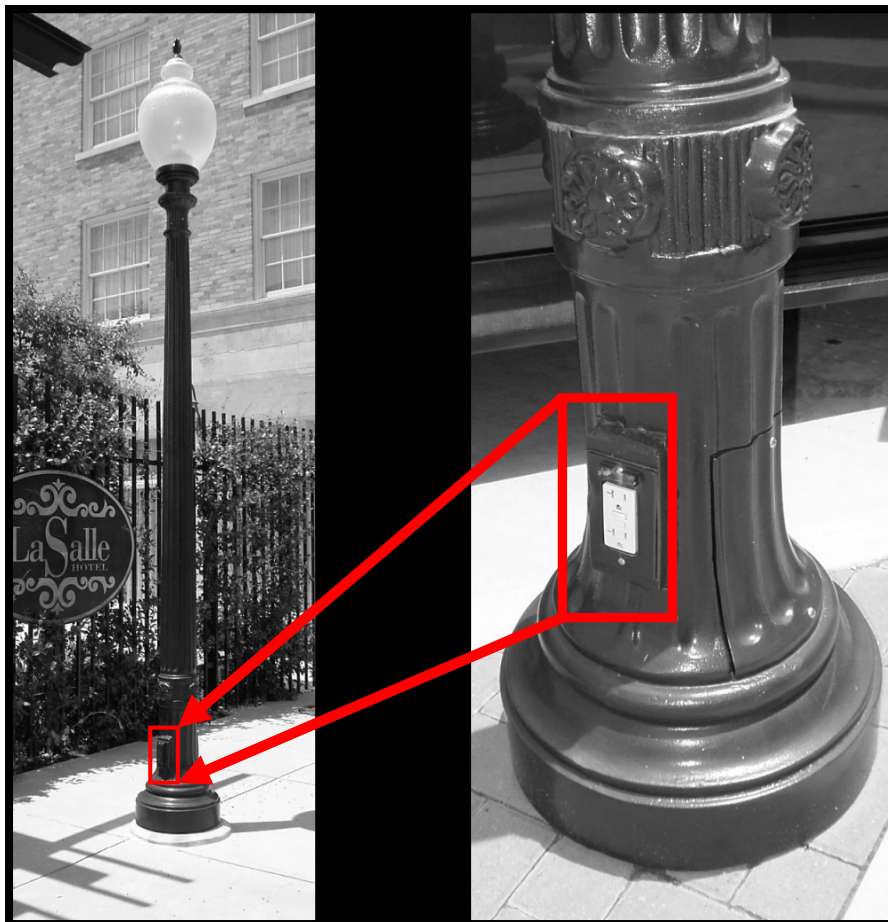
Illustration 6-33 Example of an Electrical Outlet place in a Downtown Streetlight
