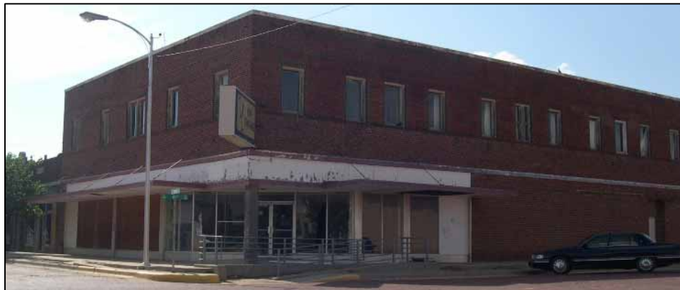
Illustration 6-16 Building with Reported Structural Problems
